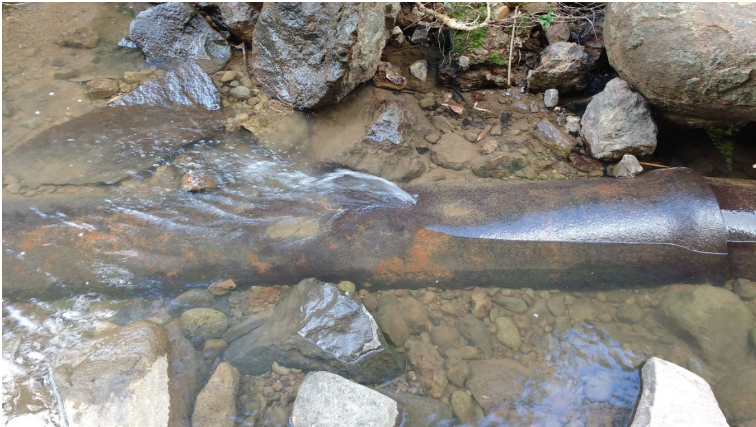
Figure 5: Sections of exiting damaged transmission pipe line (2017)
