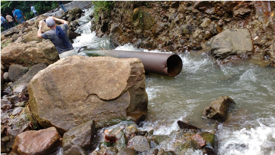
Figure 3: Damaged and displaced steel transmission pipe (2017)
