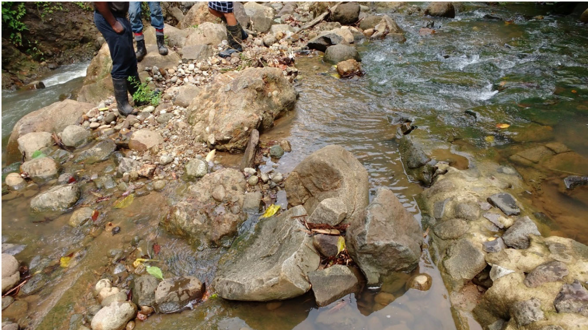
Figure 4: Damaged intake structure (2017)
